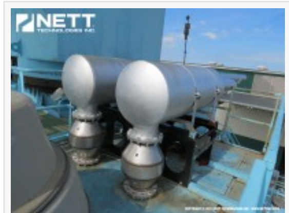
Photo of a Diesel Oxidation Catalyst(DOC)system used on a JAXPORT crane.
