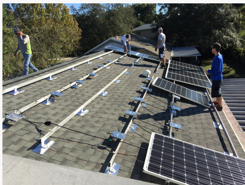
MC2 Solar's Residential Solar Panel Installations
