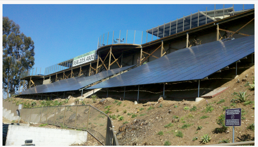
Ground-mounted solar at Soltera Ecoluxury Apartments
