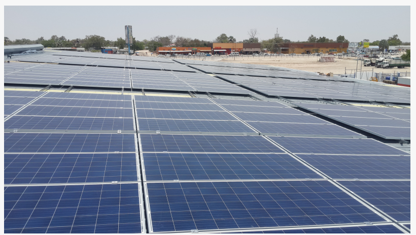
100kW of Canadian Solar Panels
