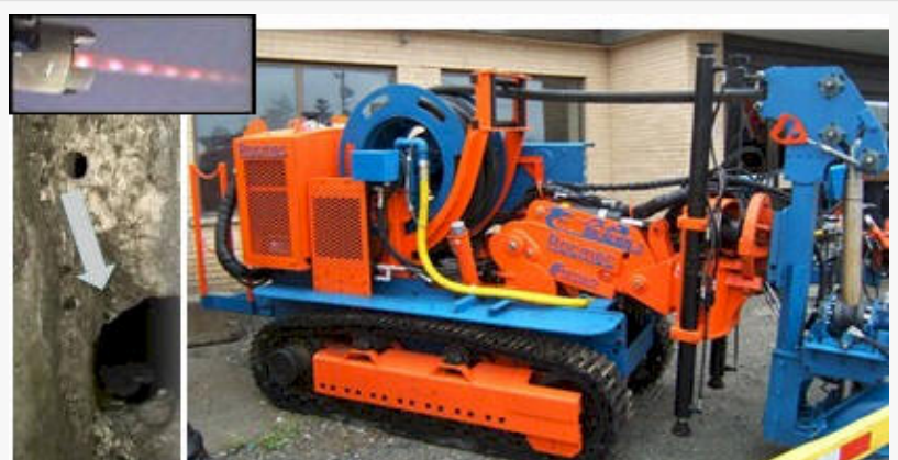
Burner able to extract up to 30 m in any direction, and image of pilot hole to 1x1m (typically takes ~8 minutes).
