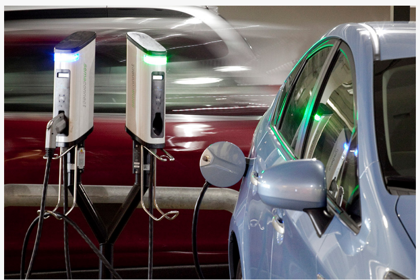
SemaConnect electric vehicle charging stations
