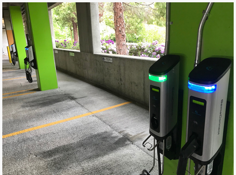
SemaConnect smart EV charging stations for commercial properties
