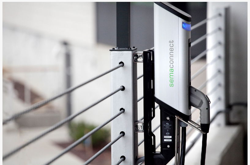
SemaConnect smart EV charging station
