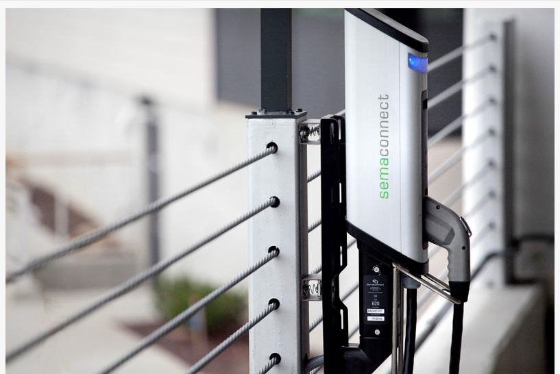
SemaConnect smart EV charging station
