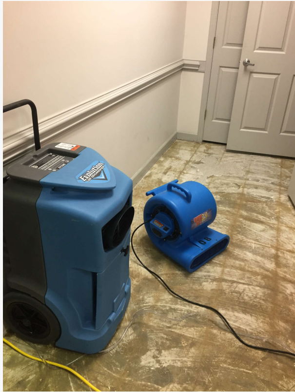
water mitigation equipment in Charlotte
