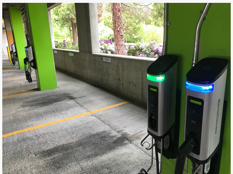
SemaConnect EV charging stations
