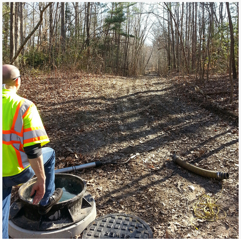
Difficult to access trunklines assessed by Focused Electrode Leak Location (FELL).
