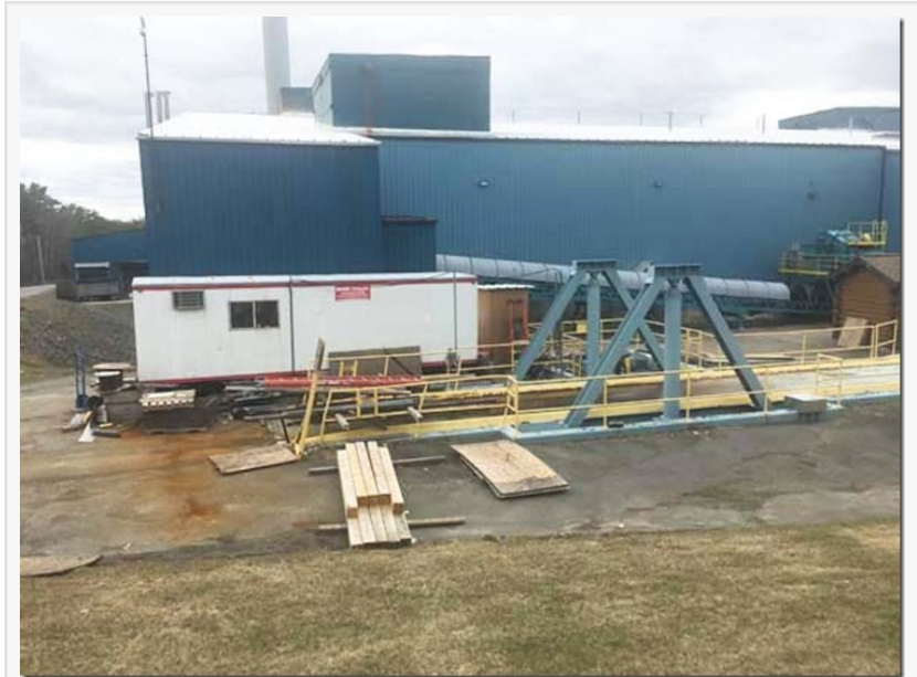
Work commences at new Maine Heat Based Phytosanitation facility for wood fuel chips
