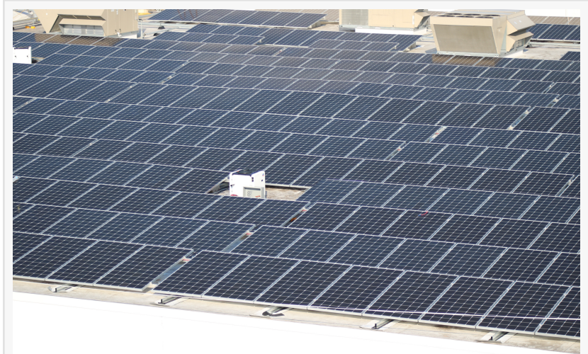
A partial view of the solar system on the roof of Designs For Vision, Inc.
