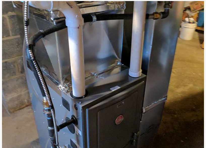
Bucks County HVAC Service
