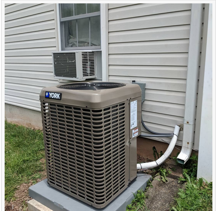
heating and air conditioning
