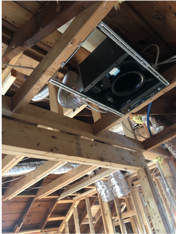
Ducted Mini Split in Ceiling
