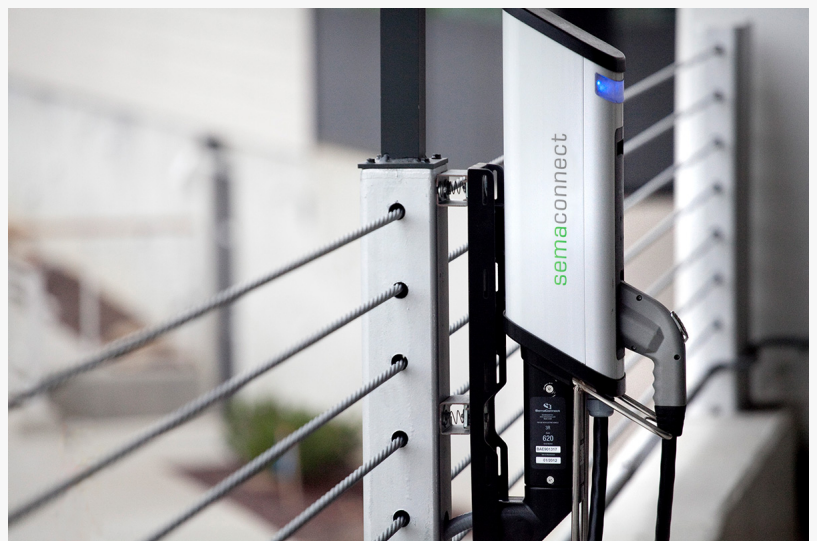
SemaConnect smart EV charging station
