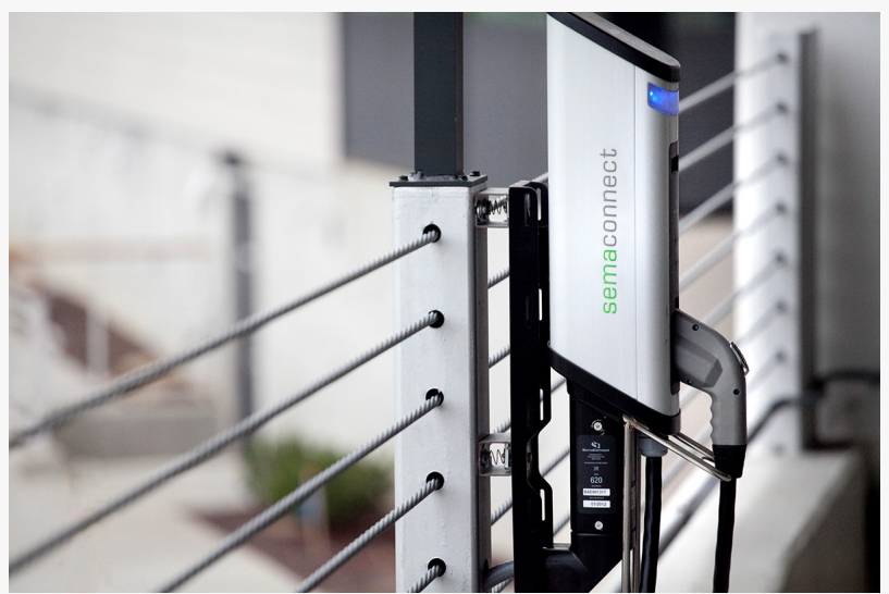
SemaConnect smart EV charging station
