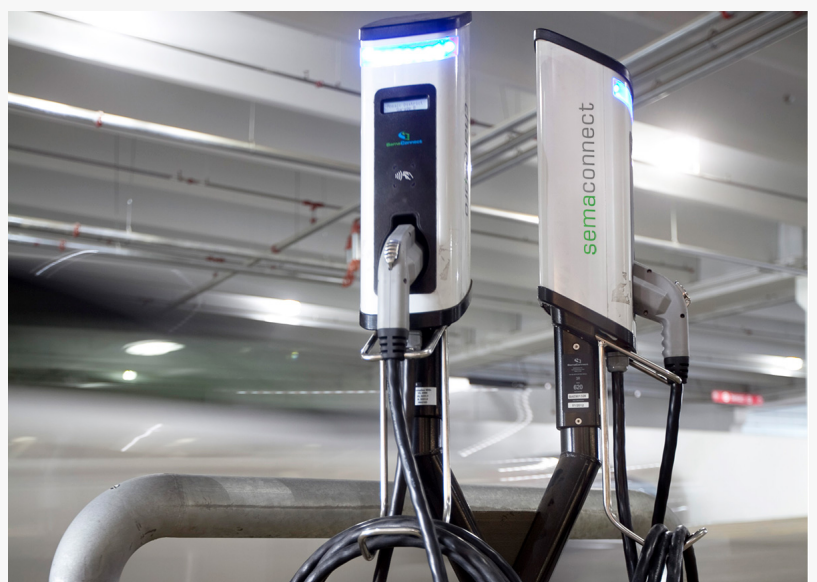
SemaConnect smart EV charging station
