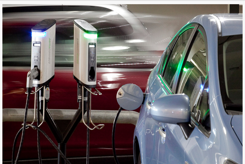
SemaConnect electric vehicle charging stations
