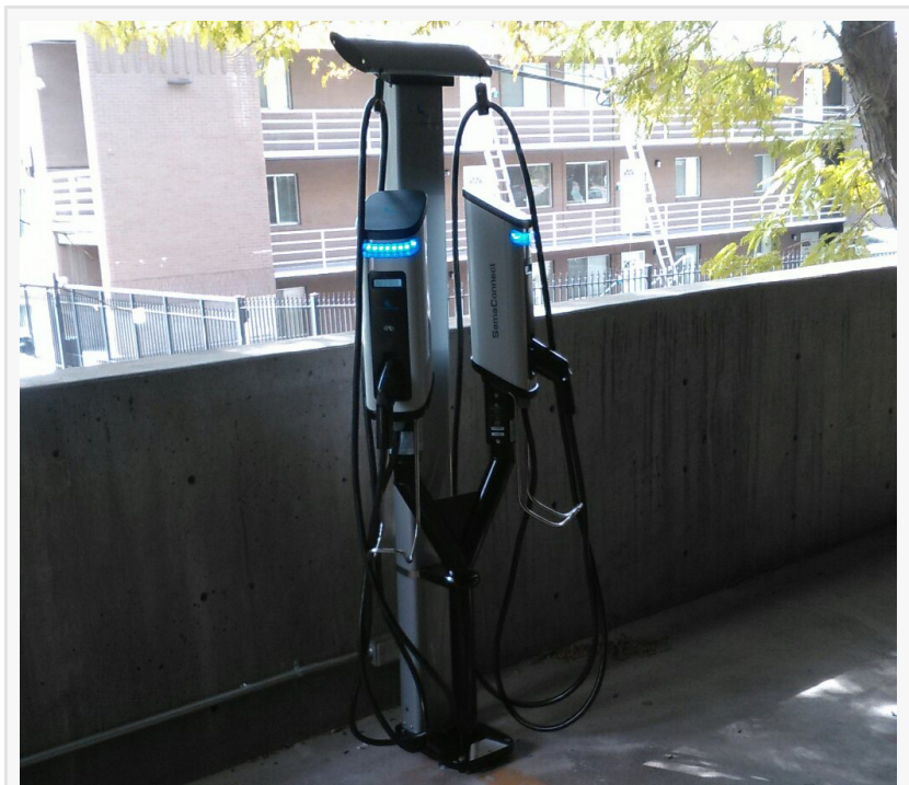
New SemaConnect EV charging stations at 420 East South Temple
