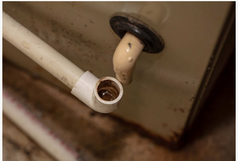
AC Drain Line Clogged Symptoms
