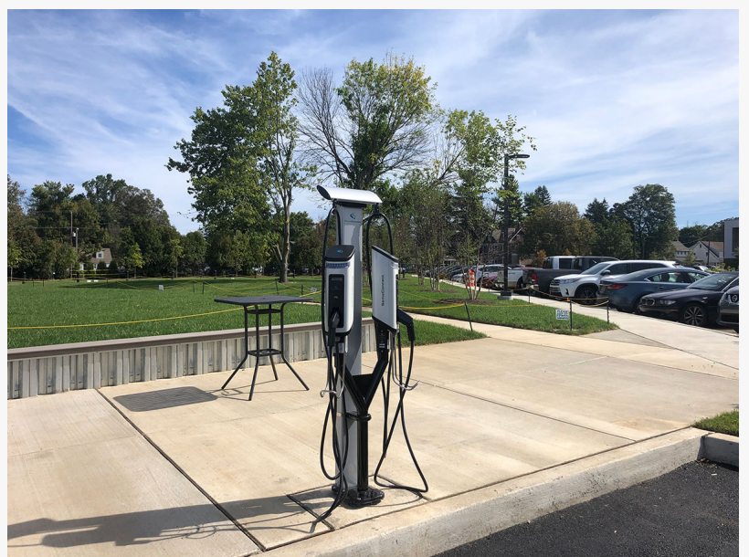
The two new SemaConnect Series 6 EV charging stations at Ambler Yards are installed outside Building 4 for employees and visitors.
