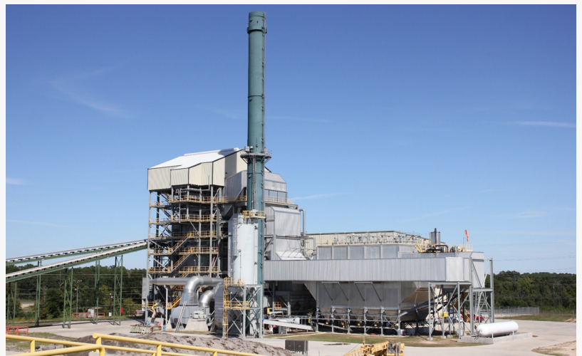
50mw Biomass Plant
