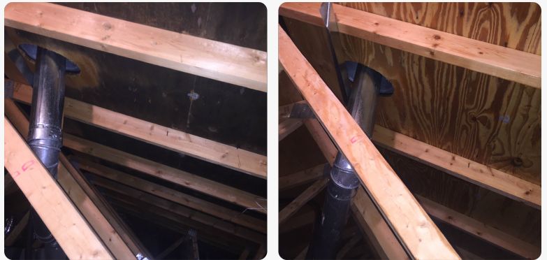
Attic Mold Before & After
