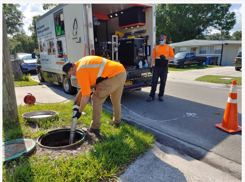
Following CDC safety measures Electro Scan is "open for business" beginning its latest inspection project in Hillsborough County's South Service Area. (ABOVE) Certified FELL operator, Dan Wise, and Regional Director, Matt Campos.
