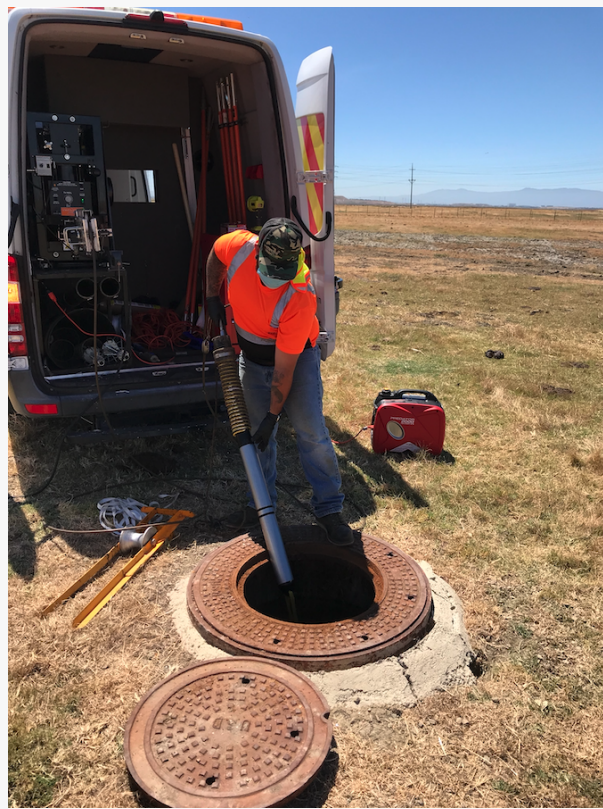
Electro Scan Operator inserts FELL probe into a Union Sanitary District large diameter sewer.
