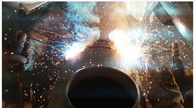
Two welders welding on the same pipe at the same time. Jackrabbit Fabrication brother-in-law SMAW welding
