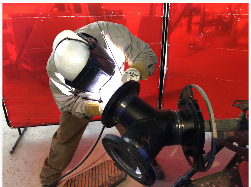
Jackrabbit Fabrication LLC Mobile Pipe Welding On Site Pipe Welding. Jackrabbit Fabrication LLC 34956 E Davis Ranch Rd Marana, AZ 85658 (520) 330-4609
