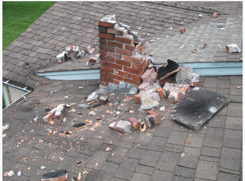
Chimney destroyed by windstorm is blown into neighbor's car.
