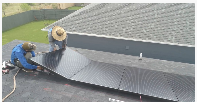
A Sunfinity installation at Whisper Valley near Austin, Texas
