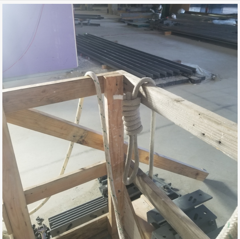
Noose at Elevator Construction Site
