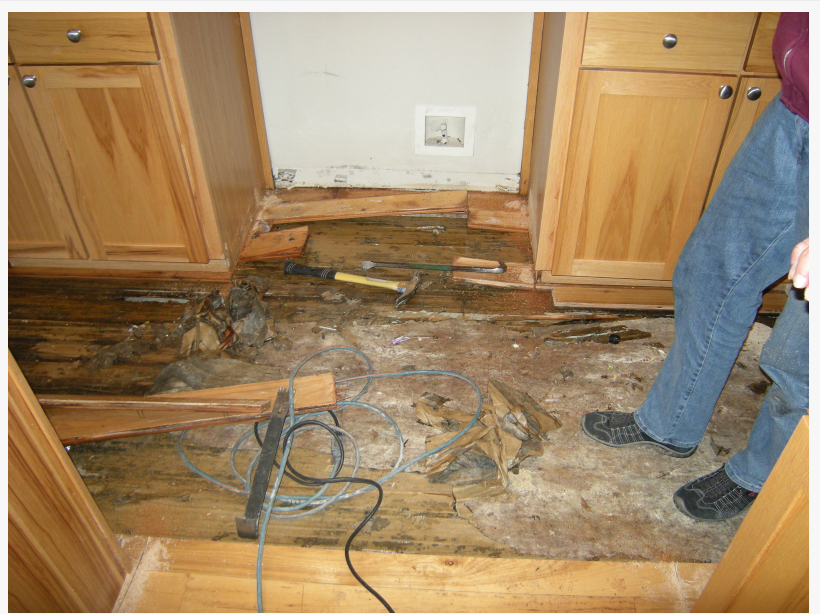
Damage to flooring from water leak.
