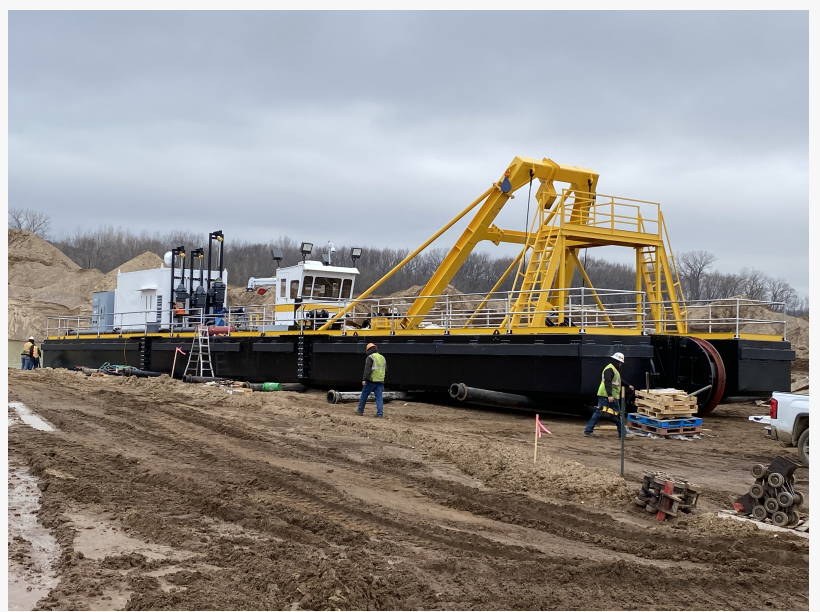
The new electric powered Cutter Suction Dredge being assembled at Legacy Materials in Booneville, IA
