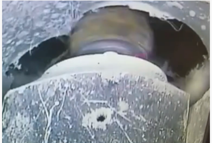
Customer service tap reconnection, frequently responsible for infiltration leakage rates greater AFTER rehabilitation, than BEFORE rehabilitation.
