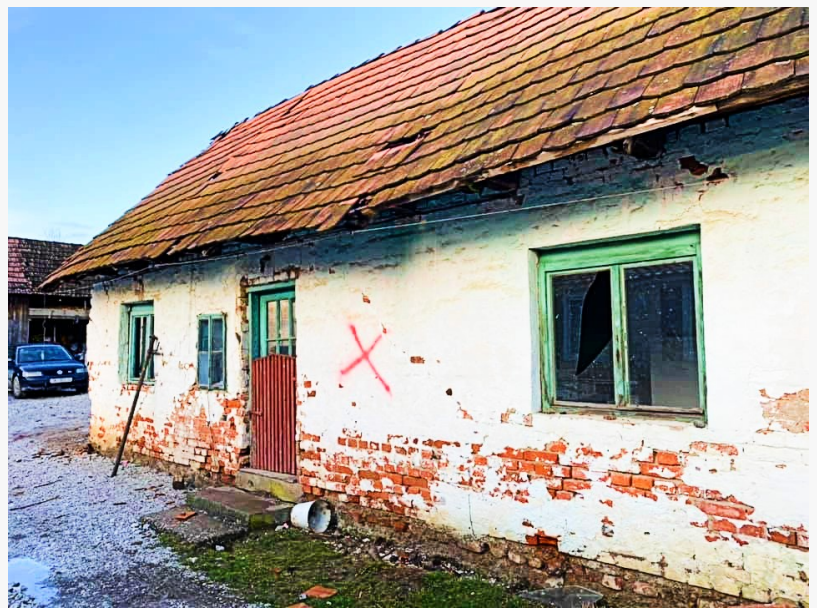
The "X" on the side of the building indicates initial inspection found the damage irreparable.
