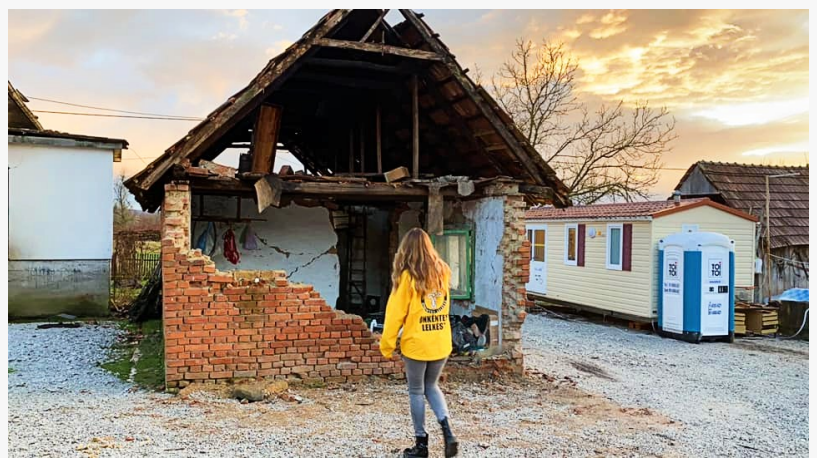
Thousands of buildings were destroyed by the Croatia earthquake leaving families at risk.
