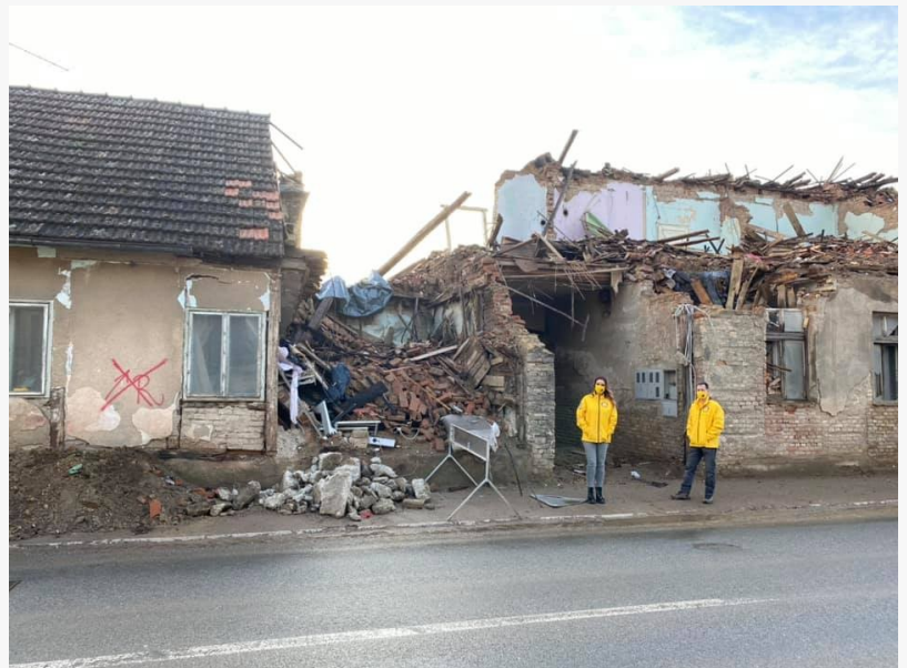
The 6.4 magnitude earthquake and 700 aftershocks have created tremendous damage.
