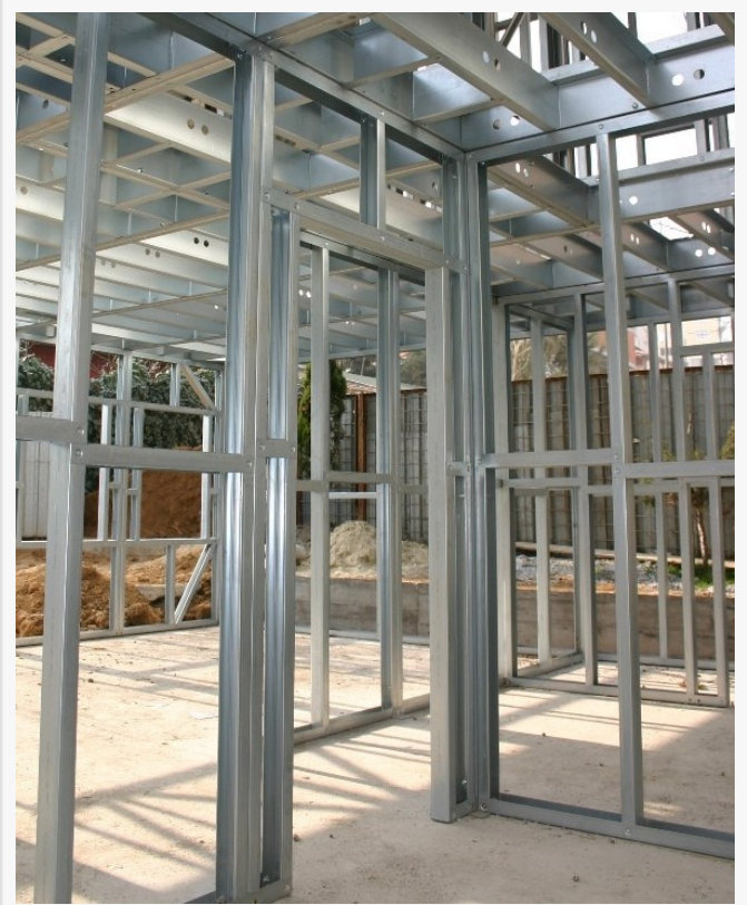
The CFS (cold formed steel) parts are assembled, creating the house skeleton.
