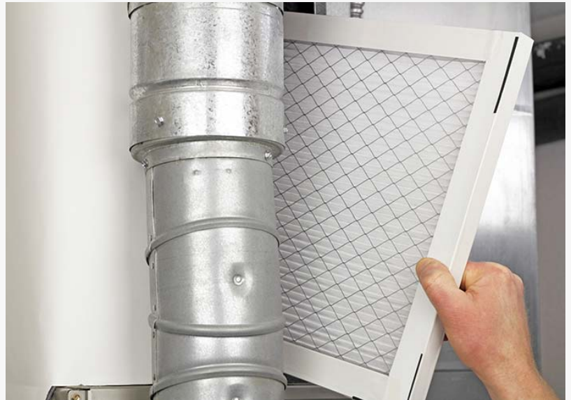
Air filter for a home in Cypress
