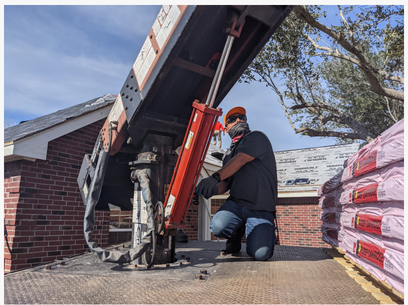
Budget Roofing Supply delivery crew member loading asphalt shingles to a residential rooftop.
