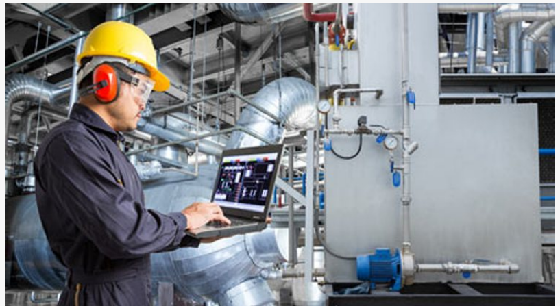
HVAC Remote Monitoring
