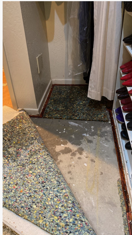
Water Damage in closet.
