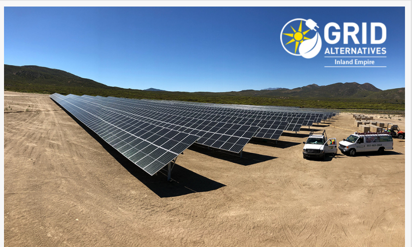
CA First Low-Income Community Solar Array
