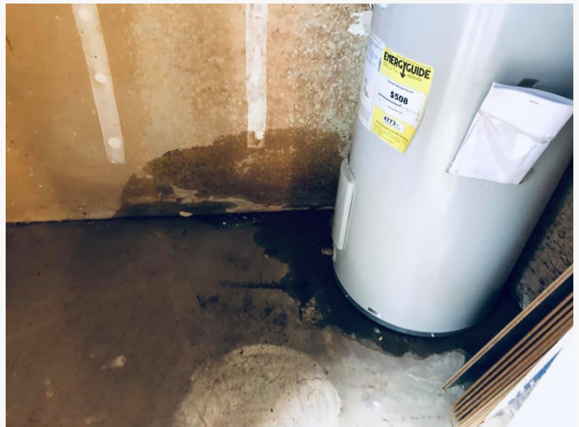
Water Heater Leak Visible Sign
