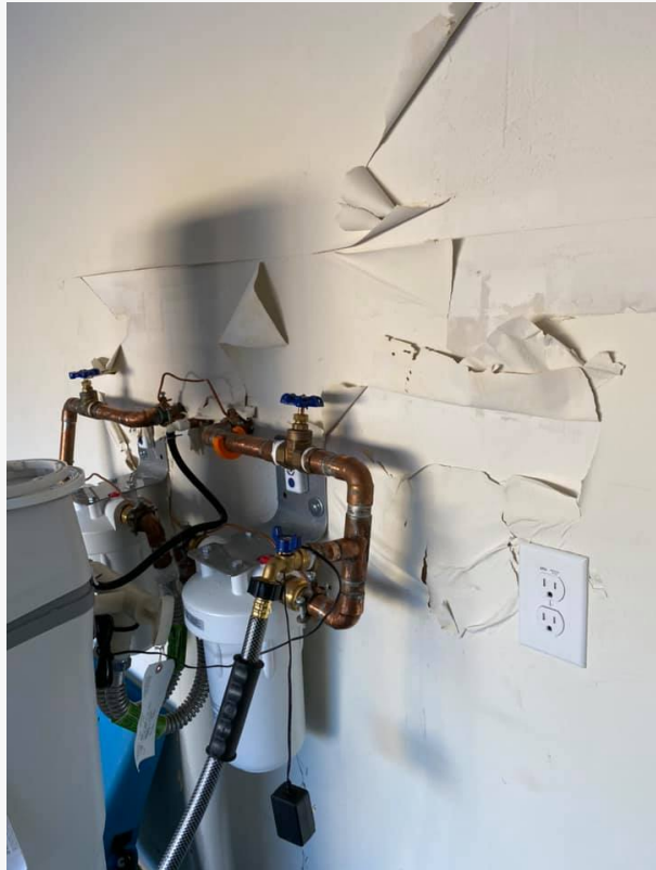
Visible sign of water damage.
