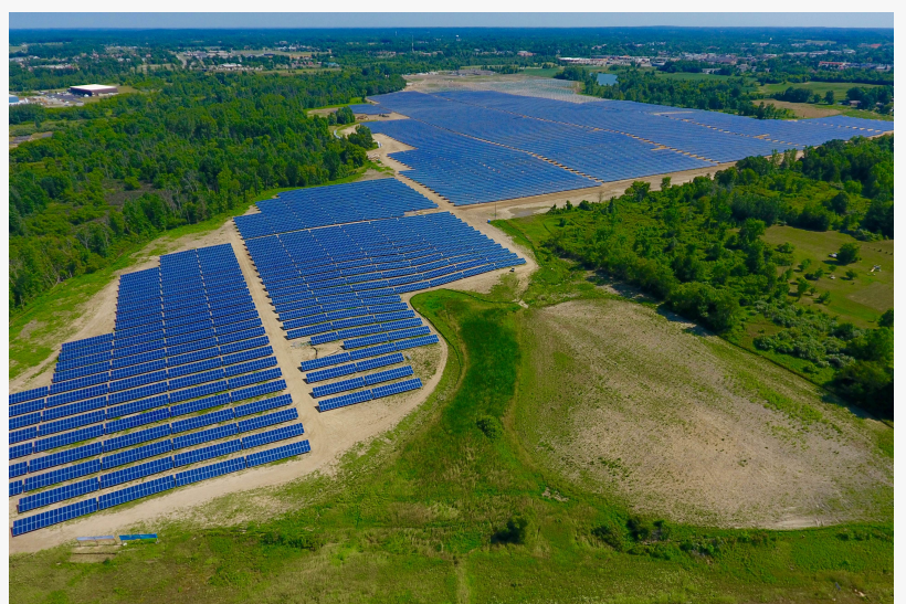
An Inovateus utility scale solar project
