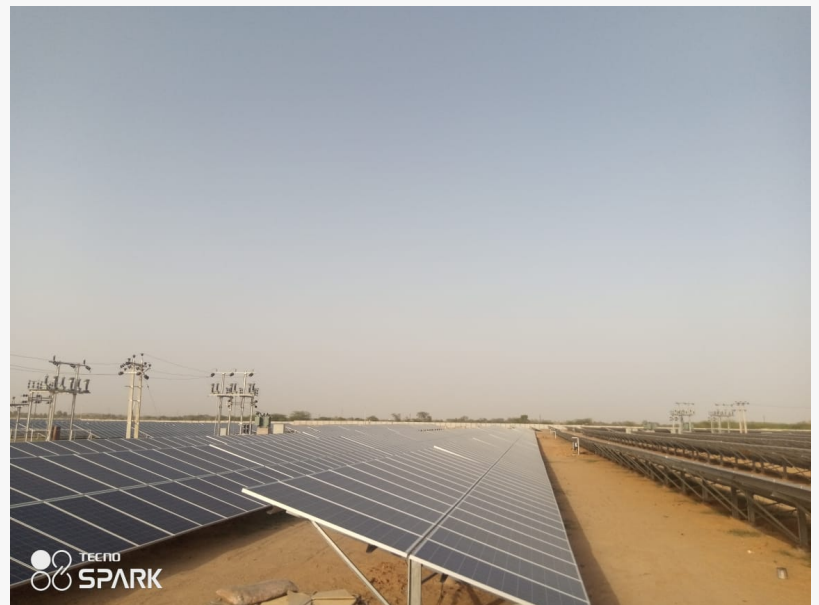
Solar panels at VGL solar plant.
