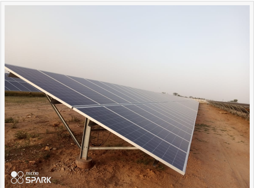
Solar panels at VGL solar plant.
