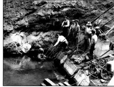
Figure 59. Construction of COPCO No. 1 in 1917 (Photo courtesy of Siskiyou County Museum, Yreka, California, P13668 OS COPCO 2).
