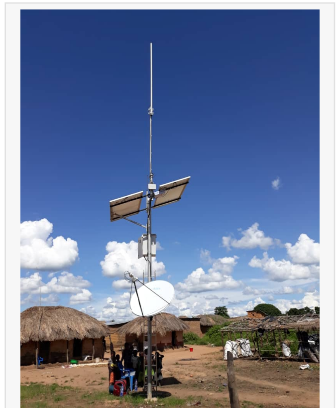
AMN Rural Base Station
