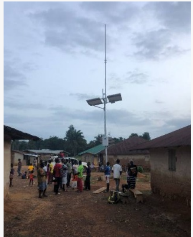
AMN Rural Base Station
