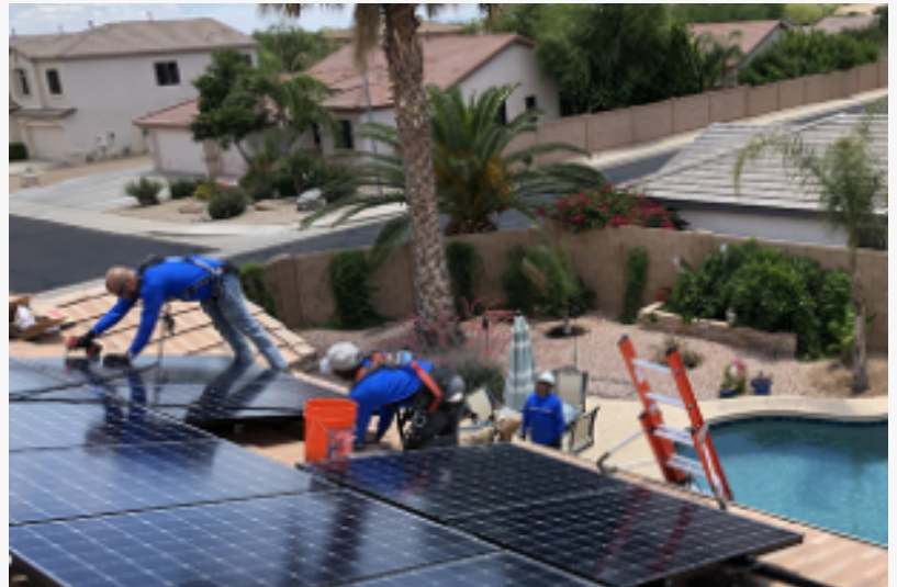
PGT Solar Installation
