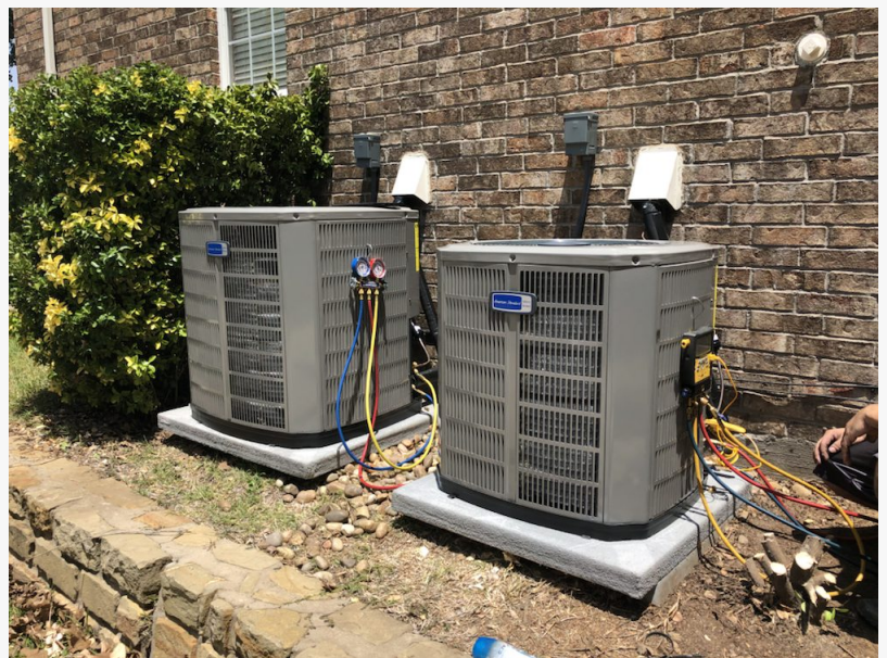
American Standard Air Conditioner Installation in Keller
