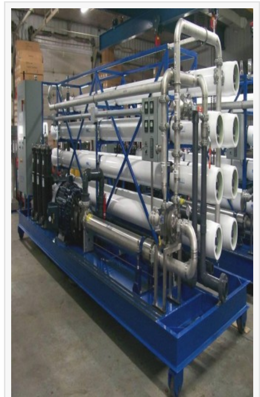
Seawater Reverse Osmosis System
